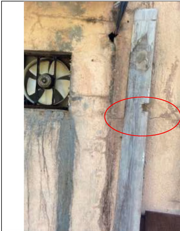
5A5-D8(2) – Moderate Crack on Wall Surface (Length:400mm/Width:1.80mm)
