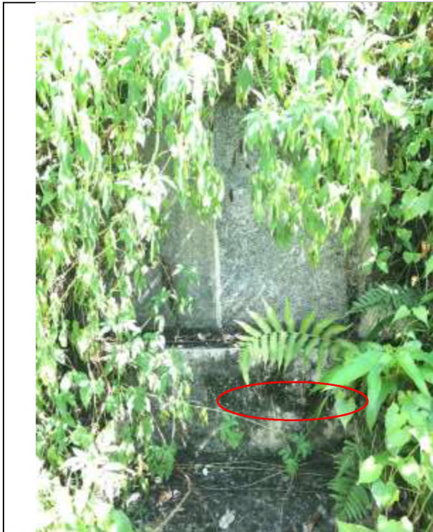
1A-D1(1) - Moderate Crack on Tablet (General View)
