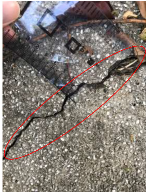
2A-D1(2) - Wide Crack on Surface (Length:1000mm/Width:2.5mm)
