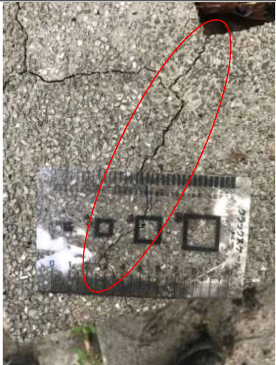
2A-D4(2) - Fine Crack on Surface (Length:200mm/Width:0.80mm)
