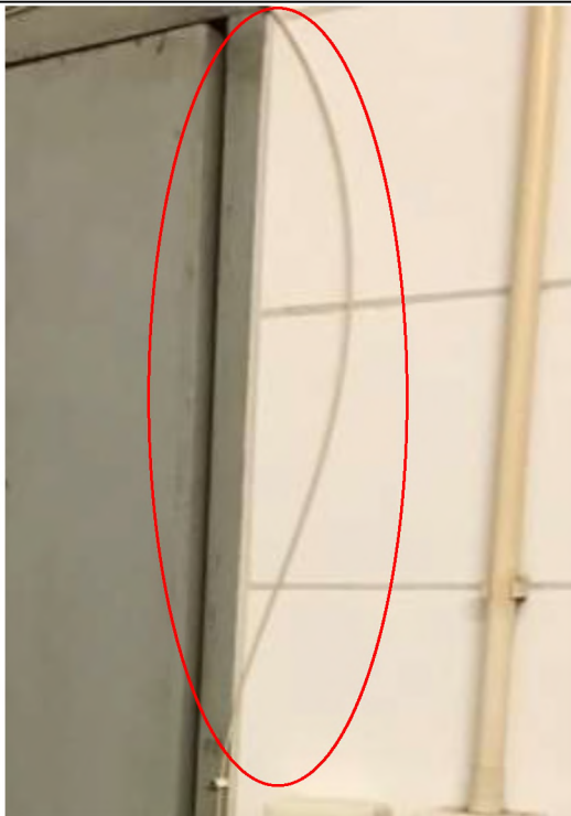
5A5-D9(2) – Moderate Crack on Wall Surface (Length:300mm/Width:1.80mm)
