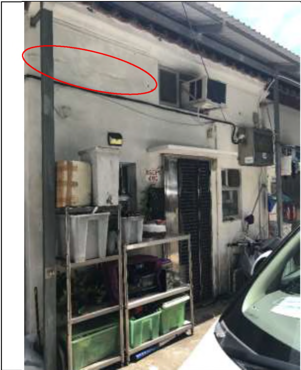
5A2-D1(1) - Crack on Surface
