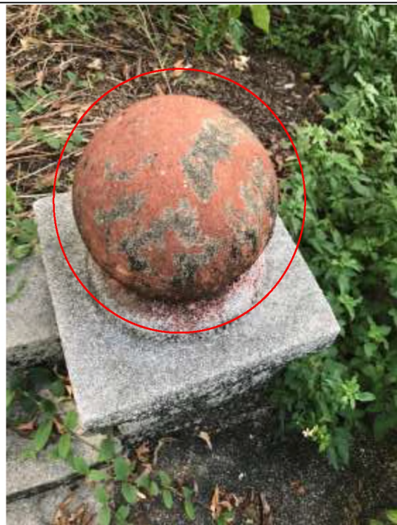
2A-D2(2) – Peeling Paint from Surface
