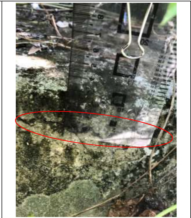
1A-D1(2) - Moderate Crack on Tablet (Length:300mm/Width:2mm)
