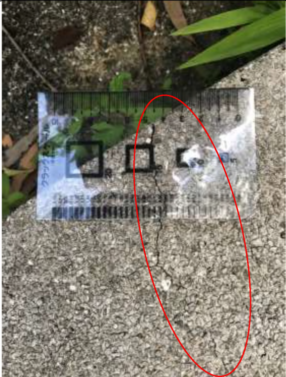
2A-D3(2) - Fine Crack on Surface (Length:200mm/Width:0.65mm)
