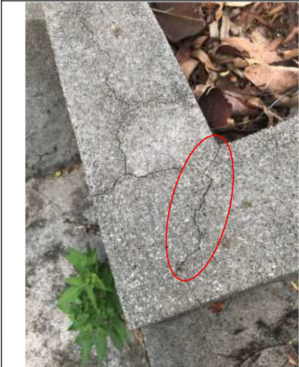
2A-D4(1) - Fine Crack on Surface (General View)
