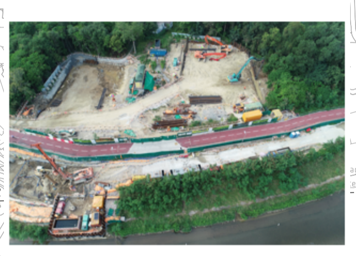
Sewage Pump Room (Portion 7), Visitor Centre (Portion 10, ELS and Pile cap) & Footbridge (Portion 9N, H-pile)
