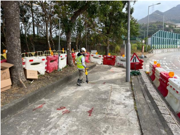
Area A: Joint Bay by CLP
